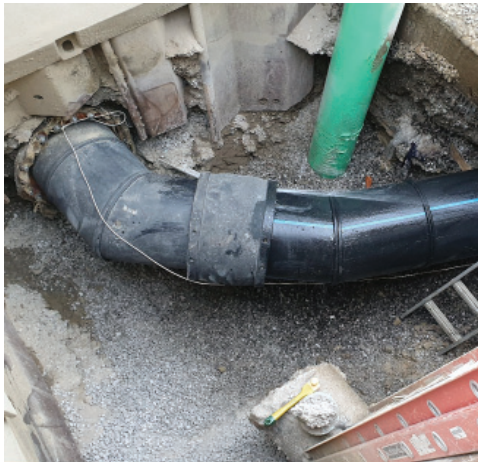
This application challenged JCM with a leaking electro fusion coupling on 22" HDPE Pipe, JCM submitted the 114 Mechanical Joint Bell Repair Sleeve style sleeve to make the repair.
