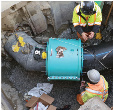
Above, the mechanical joint followers are installed on the left side of the fitting and technicians finish up the installation by installing and tightening the mechanical joint follower bolts on the right side.
